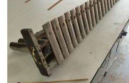
Removing the bars revealed years of deterioration on the bar rails and end caps.
